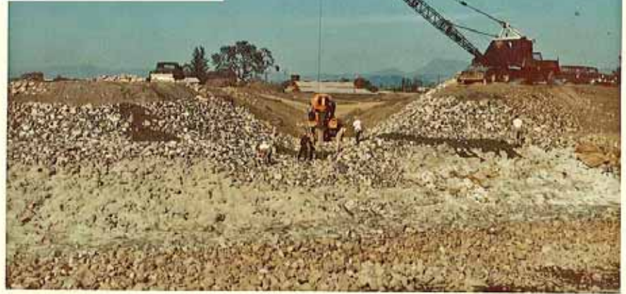
Trench excavated for 60" CMP side inlet at Willowside St. showing high water table
